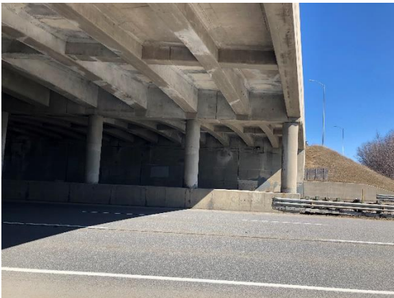
Image 5: View of the bridge soffit from the south side of the structure
