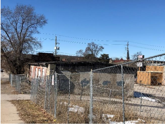
Image 7: Looking west towards the remains of the interior of the first storey of the former mill building at 69 Ainslie Street South from the street.
