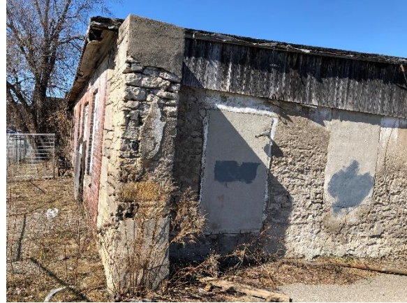
Image 8: Detail looking northwest towards the remains of the interior of the former mill building at 69 Ainslie Street South from the street.
