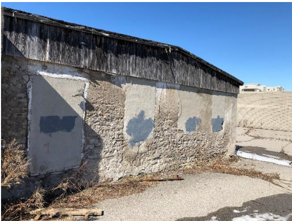
Image 5: Looking west towards the remains of the interior of the first storey of the former mill building at 69 Ainslie Street South from street.
