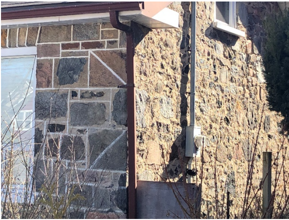
Image 15: Detail view of the transition from cut ashlar stone to rubblestone, looking north.
