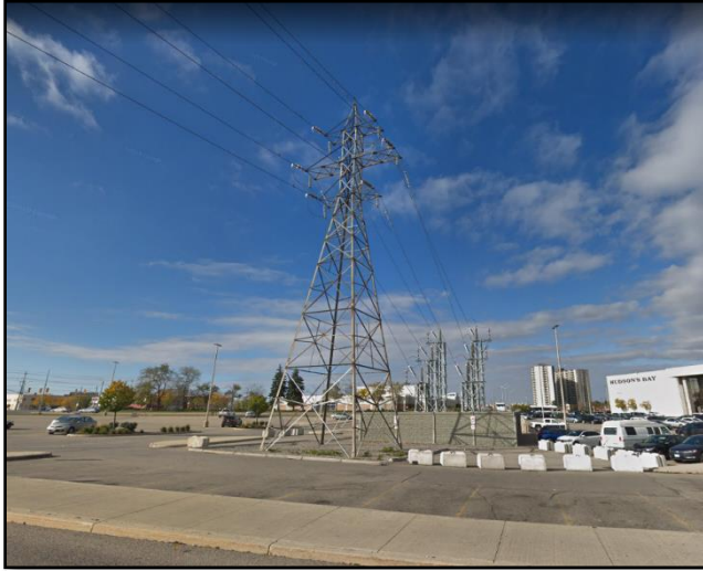
Figure 5-25: Hydro One Substation
