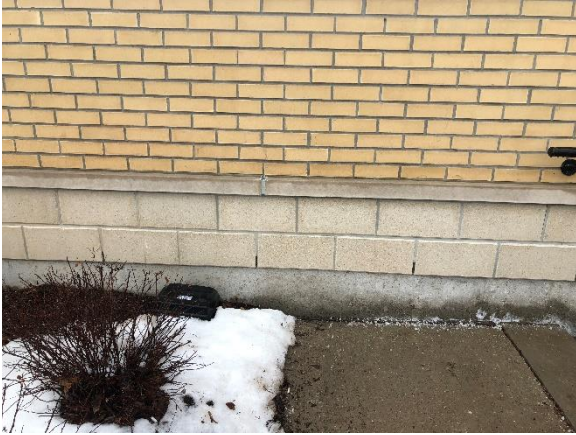
Image 15: Detail of the foundation on the west side elevation of the addition
