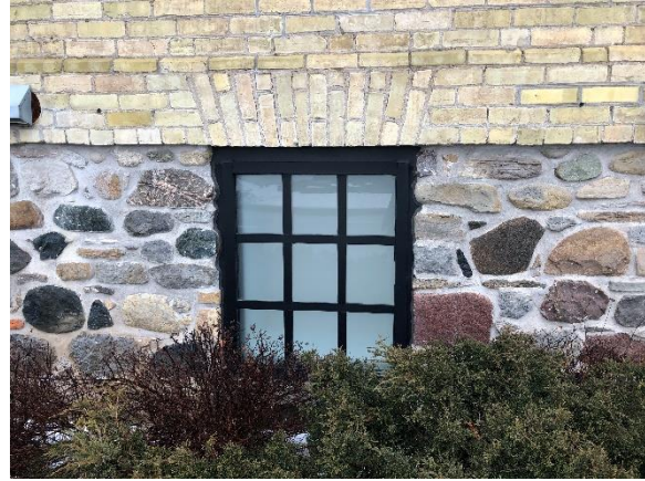
Image 16: View of a basement window opening on the west side elevation of the former Pine Grove Schoolhouse
