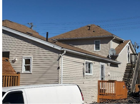
Image 12: Looking northwest towards the rear elevation of 41 Kerr Street from public walking path.
