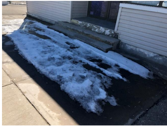
Image 8: Detail view front elevation foundation and porch steps to entranceway, 41 Kerr Street, Cambridge, ON.
