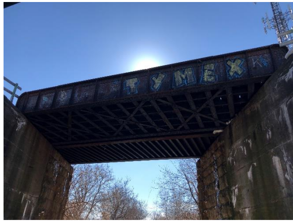
Image 13: View of the middle (foreground) and south (background) bridge decks, looking south.
