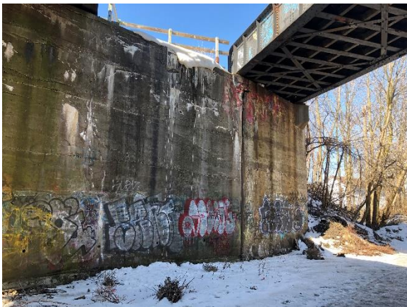
Image 6: View of the west abutment, note the expansion joint under the bridge deck.
