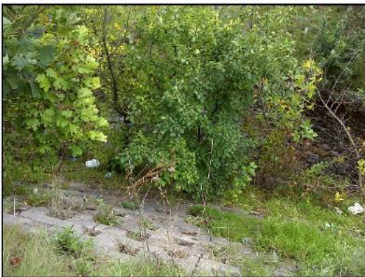
Mill Creek: Hardened bank adjacent to pedestrian trail (proposed LRT), in between Kerr Street and Main Street.
