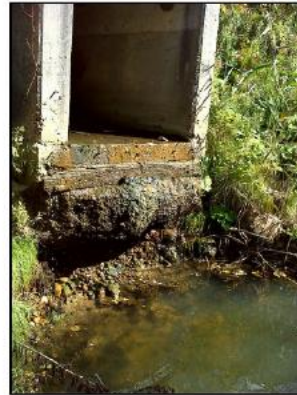
Tributary of the Grand River (North Creek): Perched culvert outlet at Hidden Valley Road, Fall 2018.
